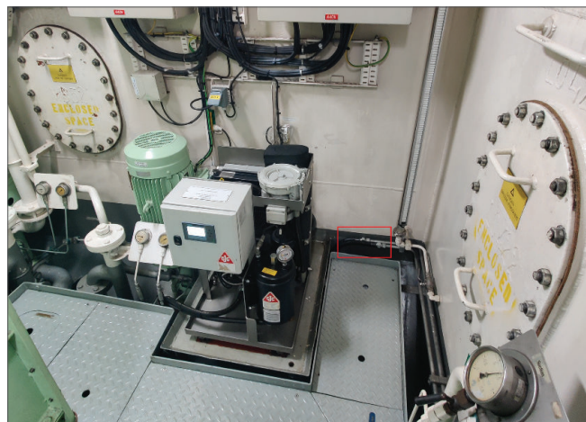
CJC® Desorber/Filter Combi Unit D5 installed on the lube oil system of the STB Stern Tube of the AHTS.
